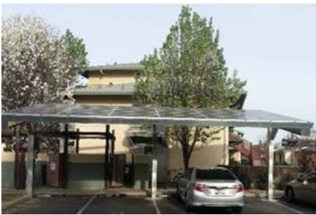
Solar Panels at Owendale Mutual Housing Community.
