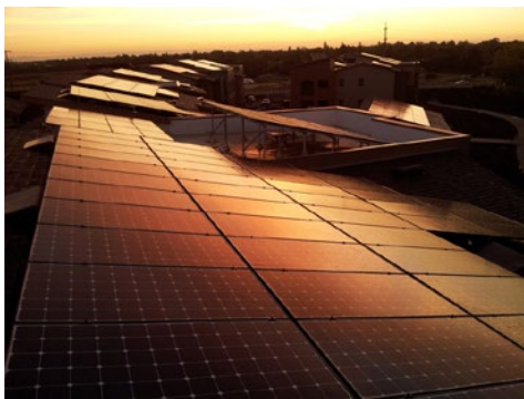
The New Harmony Mutual Housing Community solar panels at sunset. Photo courtesy Frank Domin Photography
