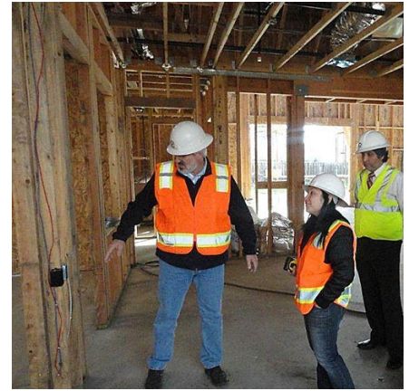
Checking out progress on the New Harmony mutual housing community, under construction in South Davis, are, from left, Bernard Keck, Sunseri Construction senior project manager; Vanessa Guerra, Mutual Housing Association project manager; and Fernando Cibrian, Mutual Housing lead organizer. Josh Sunseri, Sunseri Construction Inc./Courtesy photo
