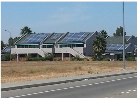
Solar panels at Twin Pines Mutual Housing Community will help residents with utility costs.
