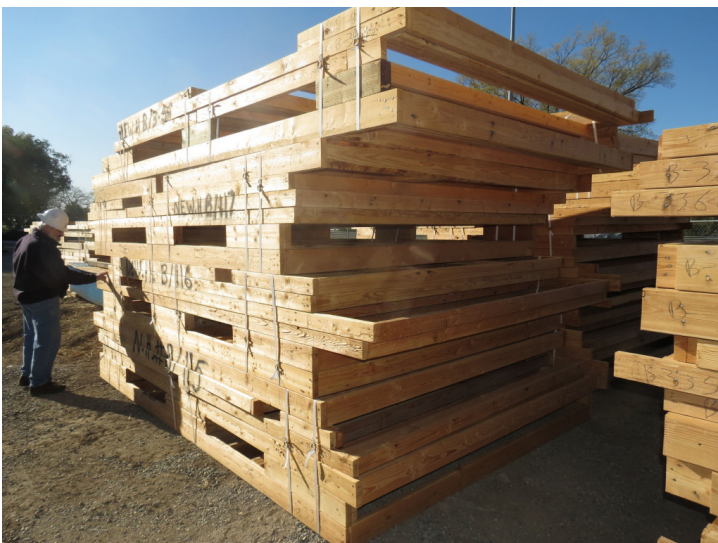
Bernard Keck, senior project manager of Chico-based Sunseri Construction Inc., examines a group of individually cut walls assembled off-site to reduce waste.
